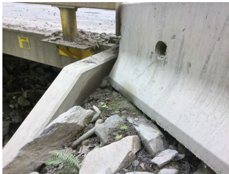
Minor fill erosion downstream left bank
