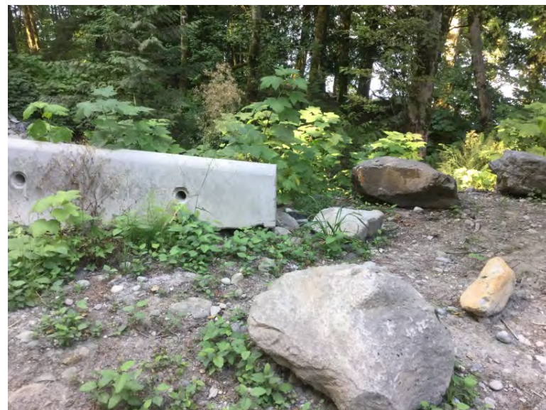
Missing downstream right bank bullnose
