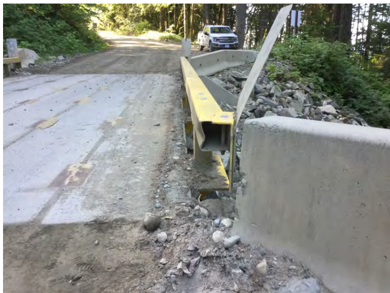
Minor guardrail damage downstream right bank
